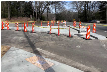
The new cross walk and medians being installed at N. Ponce and Ponce.
